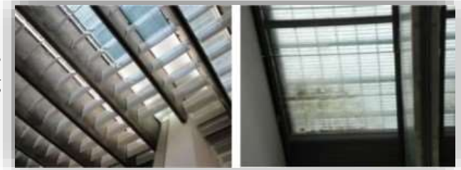
(Figure 3.21) Problems of Skylight
