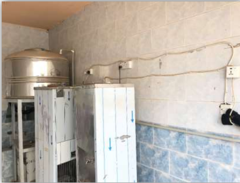
Artificial Heating and Energy Generating System
